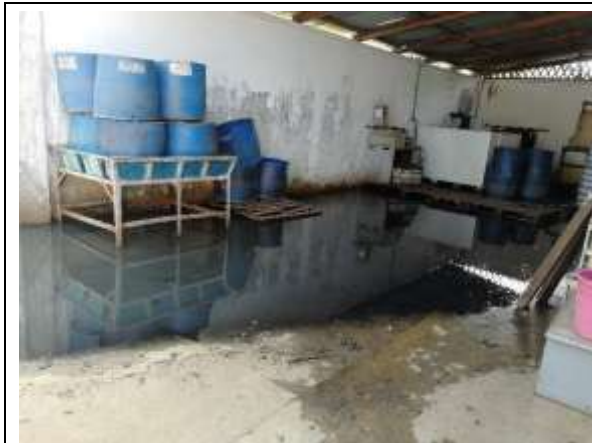
Current unsafe treatment location
